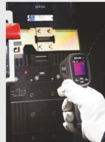
TG165 high voltage thermal reading
